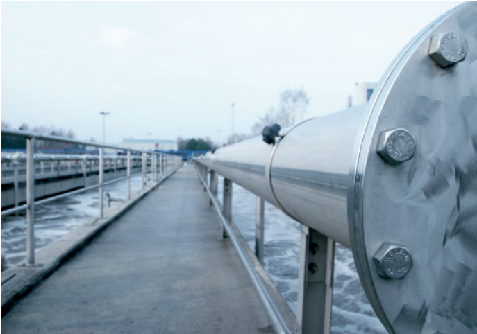
Aeration basin of a wastewater treatment unit
